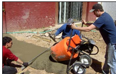
St. Charles Borromeo, Skillman, New Jersey, high school students pouring sidewalks for the hall
